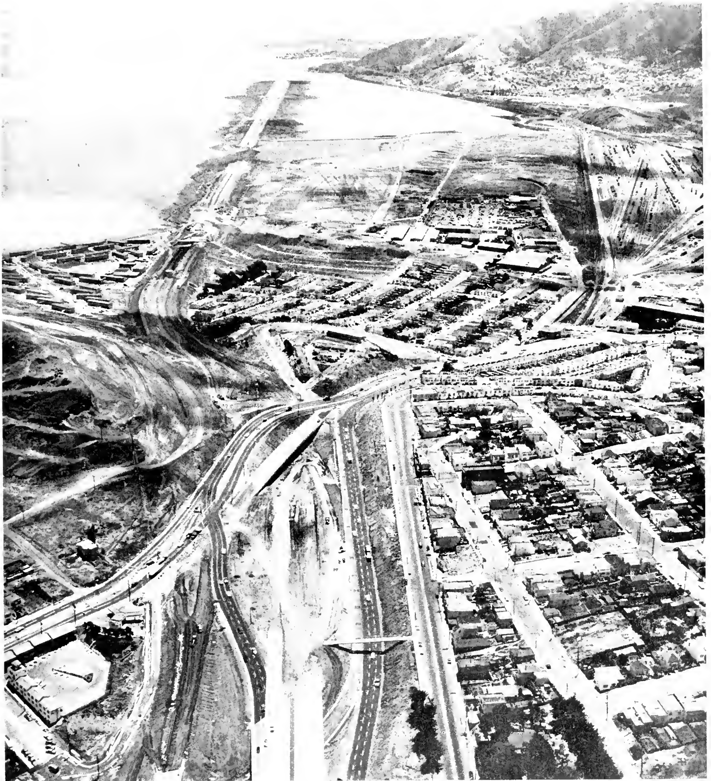
Construction operations on Bayshore Freeway from Third Street Interchange in foreground. Looking southerly along open water fill toward Sierra Point. The Division of Highways is advertising for bids on a project which will complete all rough grading and structures required to close the overwater gap on the freeway.
